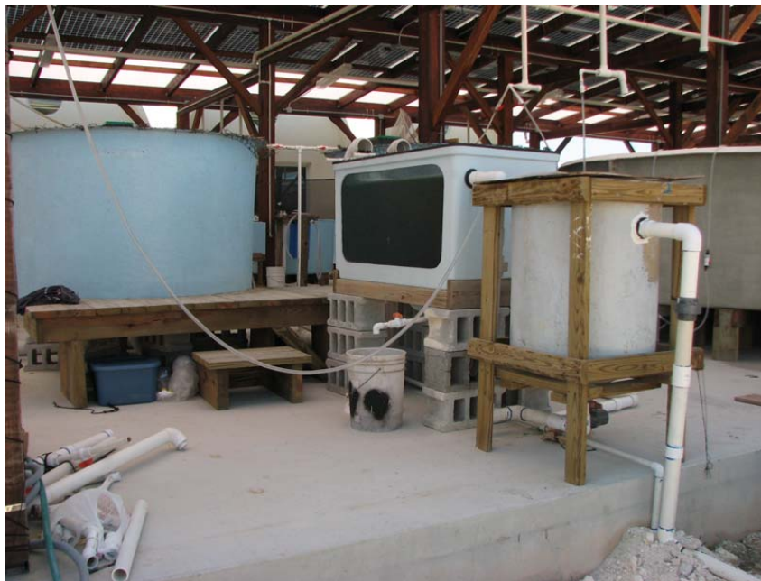
The Tilapia fish tanks, the settlement tank, and the biofilter are all housed in the Wege Center for Sustainable Fisheries – the world's first solar-powered hatchery and wet lab center.
